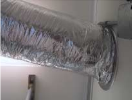
Duct To Generator Room
