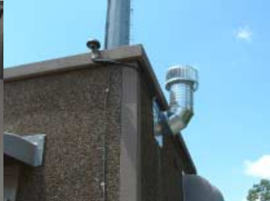
Aura Vent In Generator Room
