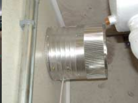
Generator Room Duct Outlet
